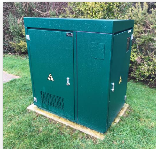
Access (Active) Cabinet
